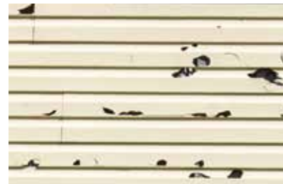
Other siding after hail
