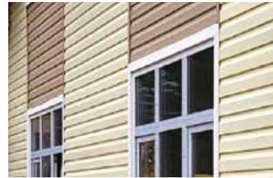
Siding Döcke after hail
